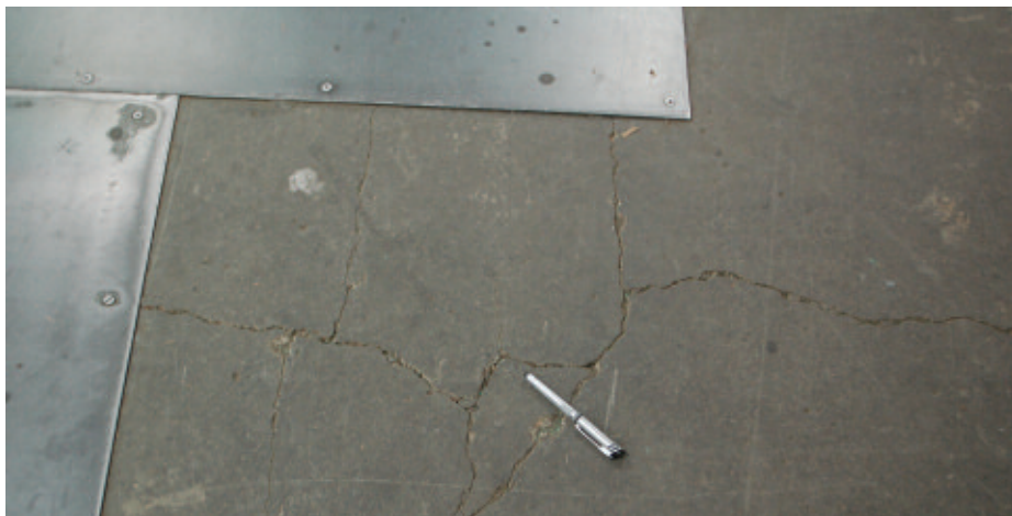
Prior to ResinDek repair, steel plate had to be attached on top of the concrete mezzanine floor so pallet truck wheels could continue to roll
